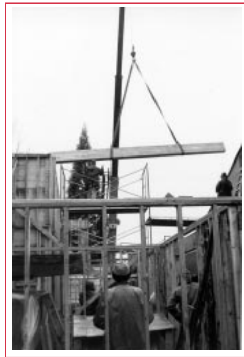
Lane Community College students get on-the-job training working on LRAPA's building remodel.
